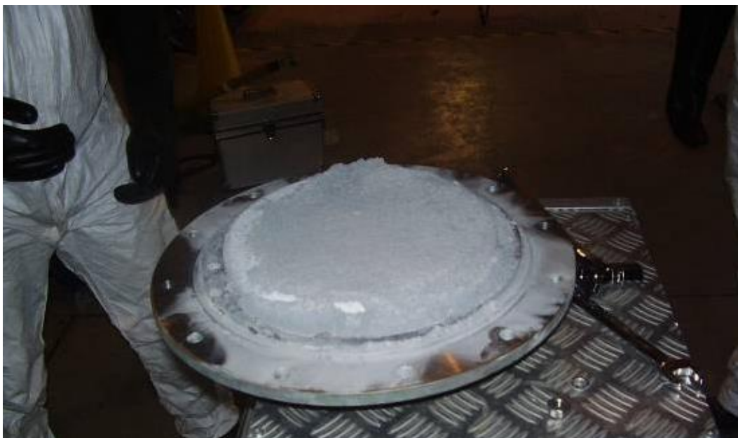
Figure 1 – SF 6 By-products contamination following arcing
