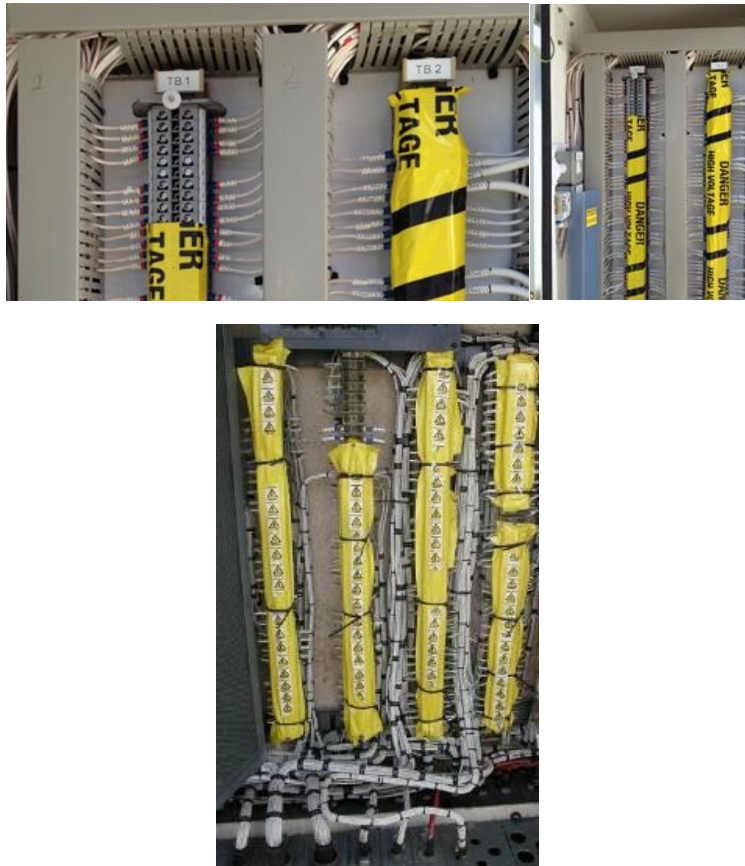
Figure A1-3 Example of screening on terminal rails
