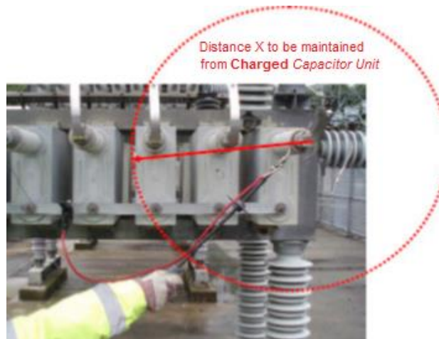
Figure 5.2.1b – Discharging single bushing Capacitor Units with LV terminal on Capacitor Rack frame
